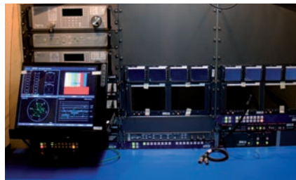
TV mobile unit installation
